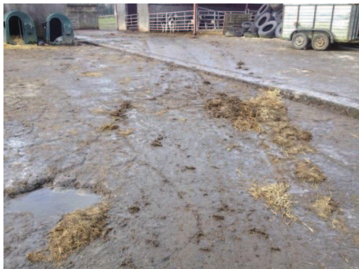
Figure 22: uneven, broken surface of yard
