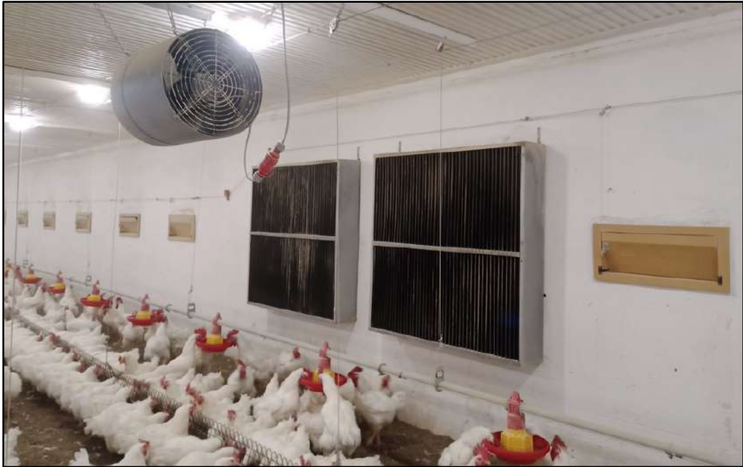
Figure 16 (above) Inside a “C technology” barn. On the wall are light traps as the inner side of the evaporating curtain and the yellow inlets. The mixer ventilator is hanging from the roof.
