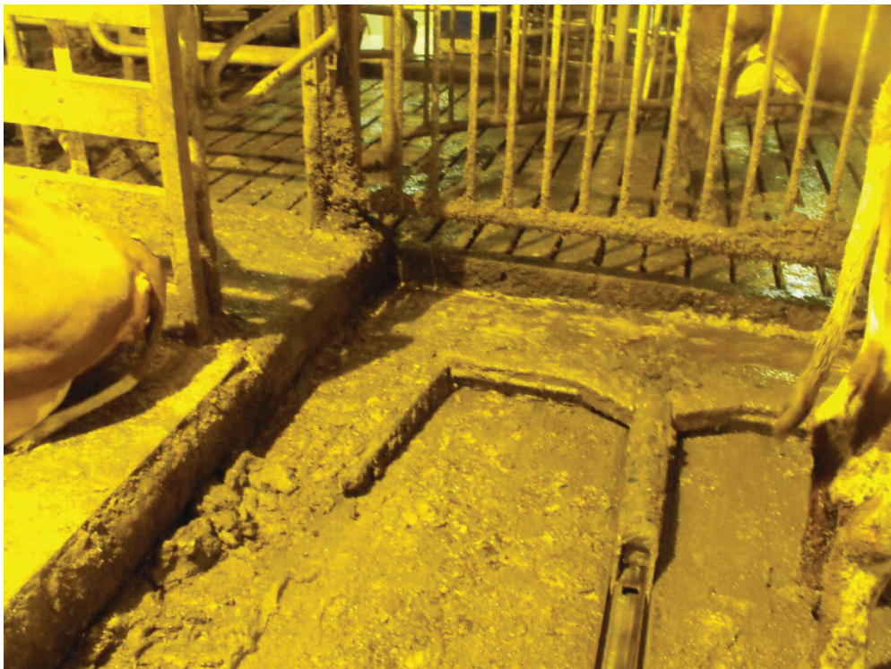
Figure 9, an unnecessary high step coming out of the sorting gate, straight onto the scraper.
